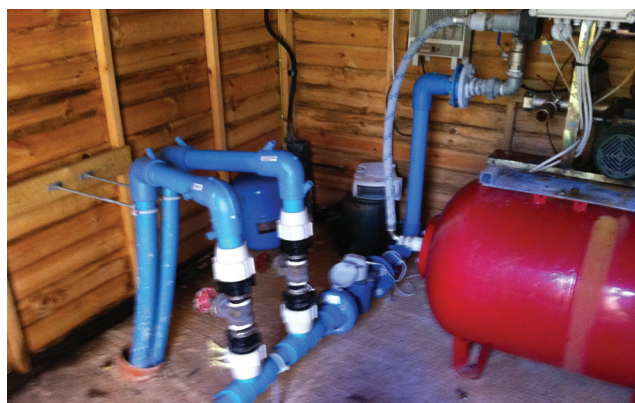
Figure 1: The customer saves $50,000 per year by using a borehole supply instead of mains water
